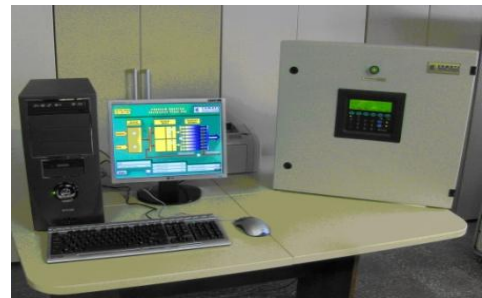
Wastewater Treatment Plant Monitoring and Control
